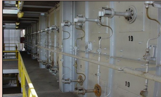
100's side wall burners
