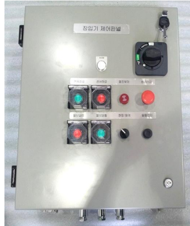
MAIN CONTROL PANEL
