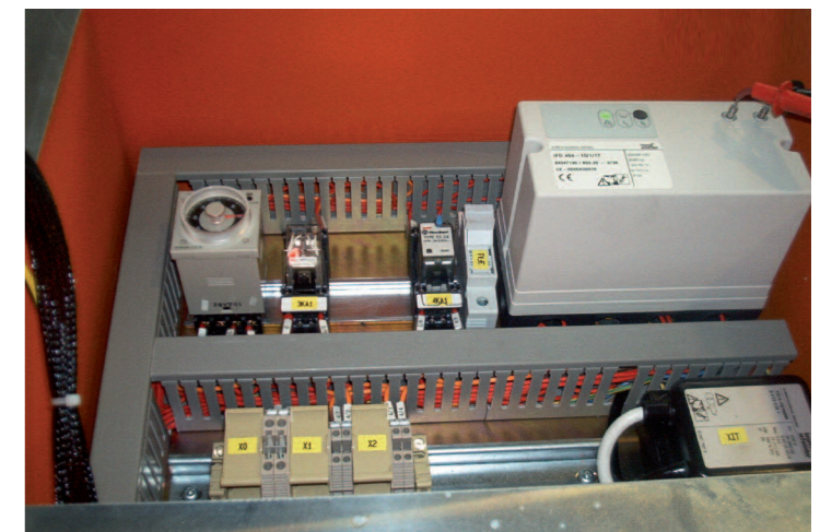
IGNITION TRANSFORMER AND IONIZATION AMPLIFIER INSIDE EExd BOX
