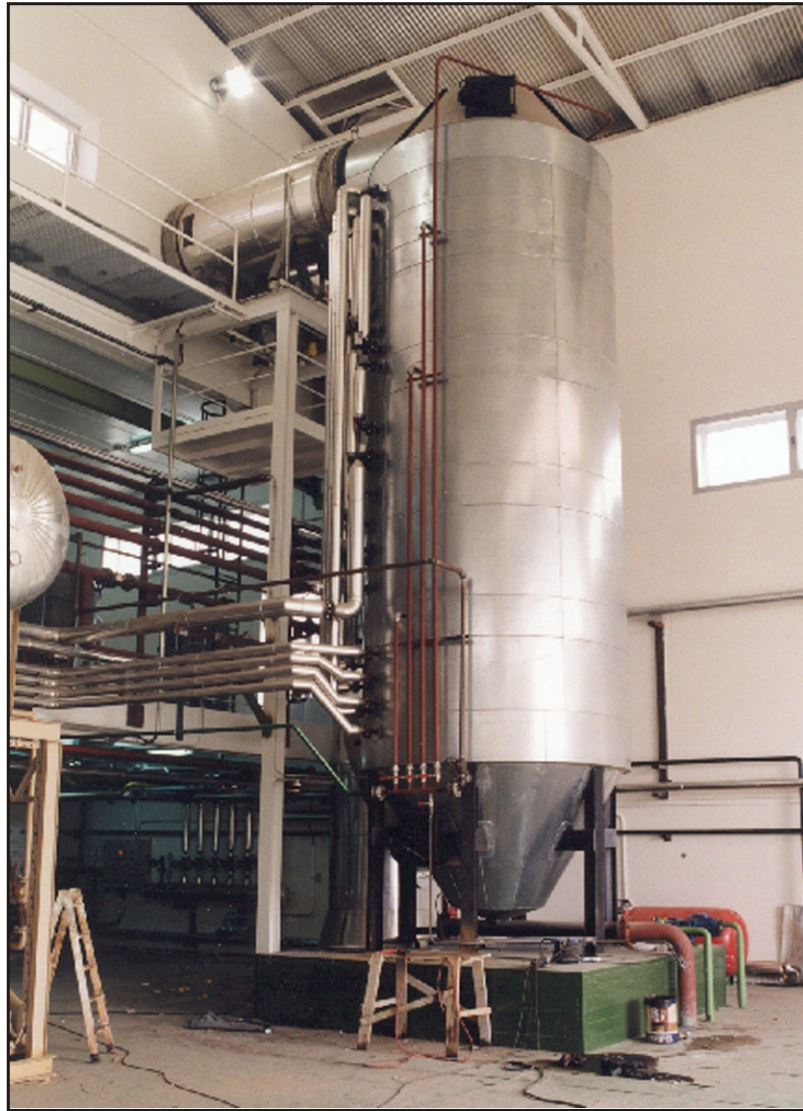
EXHAUST GAS BOILER 4 t/hr. STEAM
